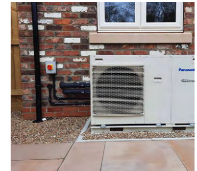
ref.14: Image showing Air Source Heat Pumps
